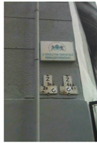
CCTV in a public space of Budapest
